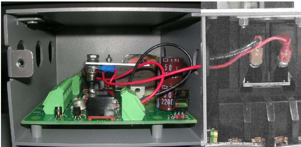
Fig 15 (New Control board with voltage regulator)
